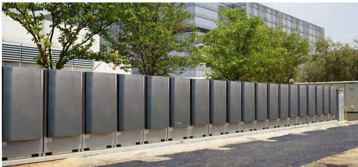
FIGURE 2.6 Commercial fuel cell installation in India
