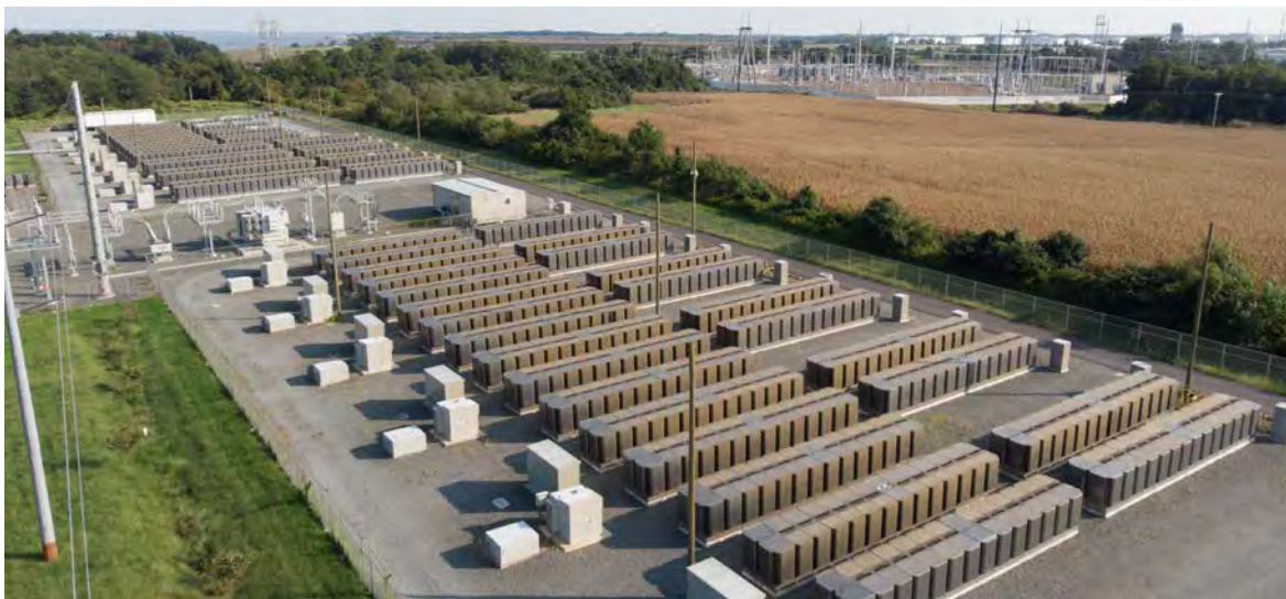
FIGURE 4.5 Utility-scale fuel cell solutions: Solid oxide fuel cell units in the US
