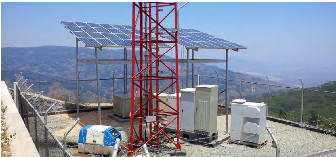
FIGURE 2.5 Fuel cells for critical infrastructure in Indonesia
