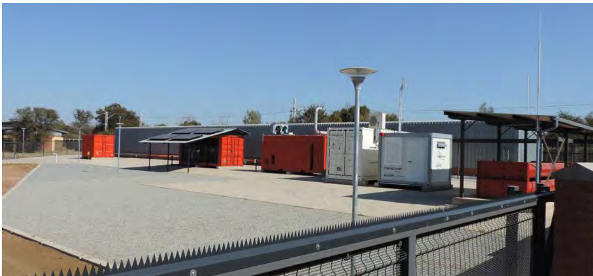
FIGURE ES.2 Hydrogen South Africa solar plus battery, hydrogen electrolysis, and fuel cell system
